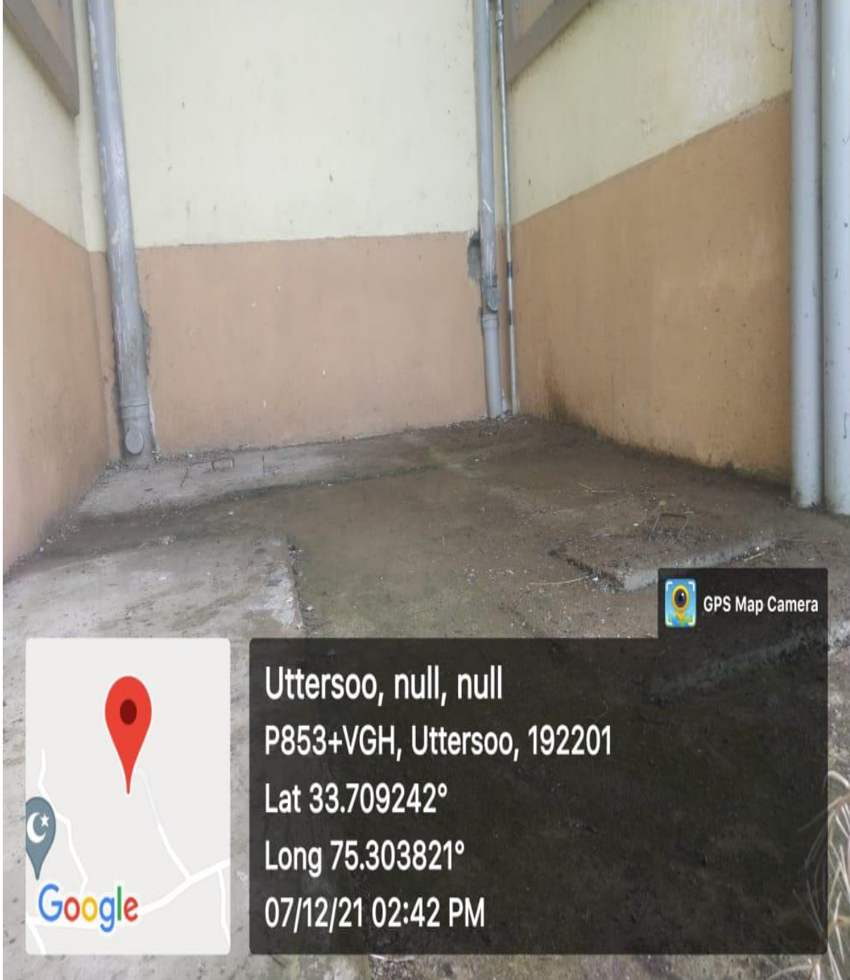
Figure 1: Liquid waste flows into covered trenches
